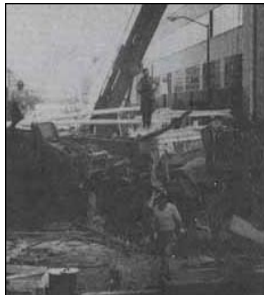
Tower Crane Collapse (Cleaning Up Debris)
